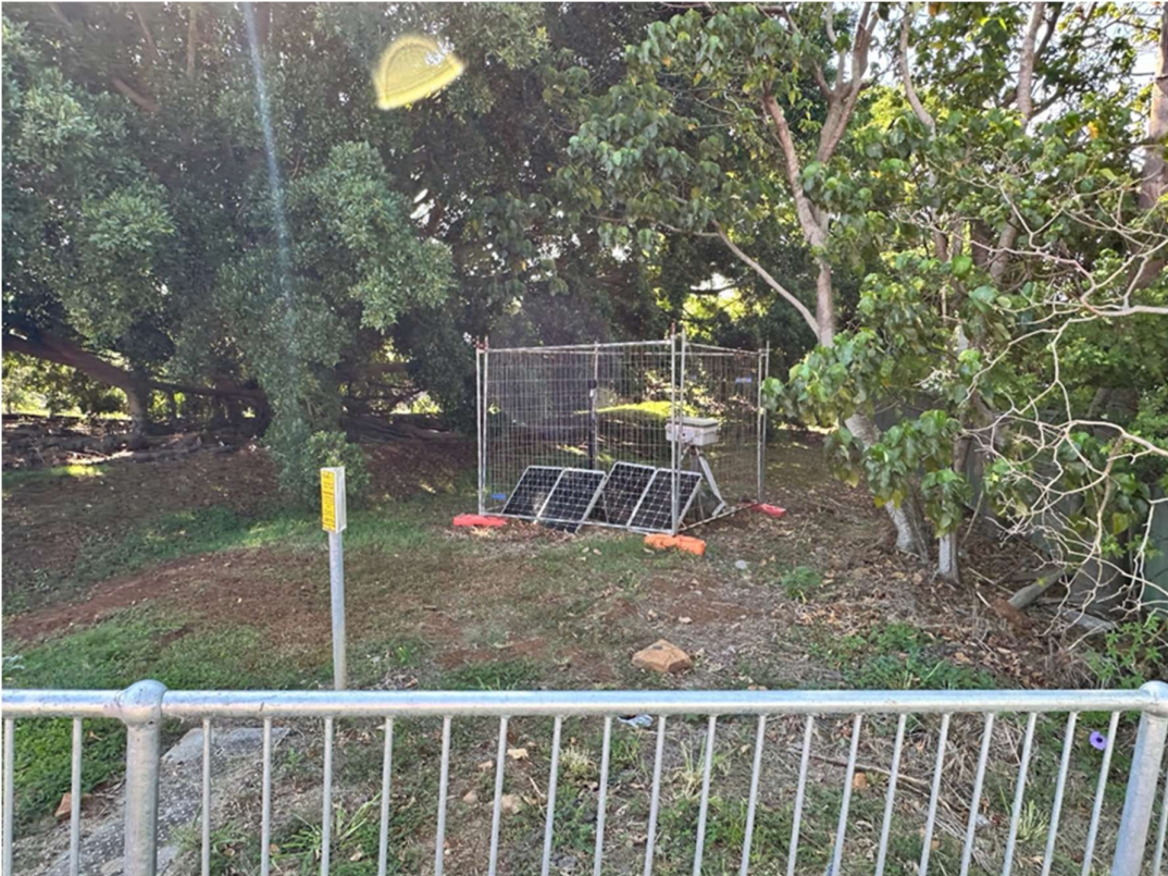
Photo 14: Noise and vibration monitoring equipment
