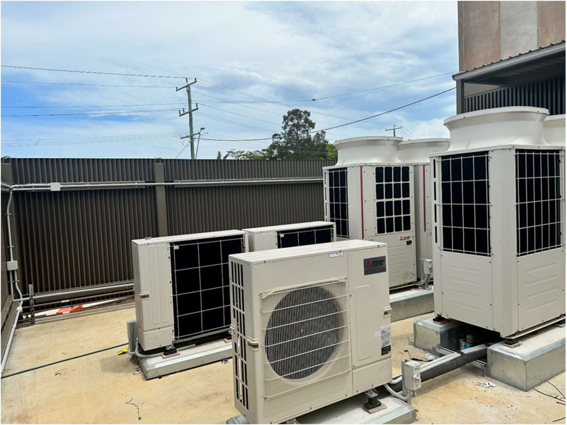
Photo 10: Health hub air conditioning units and acoustic fence
