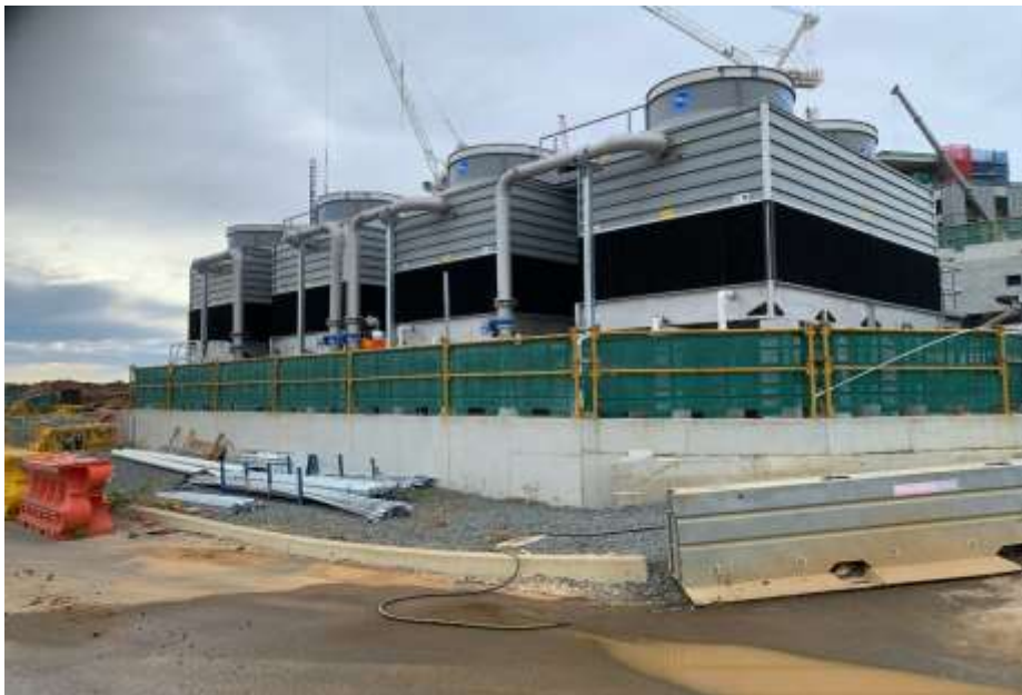
Photo B1:2 Mechanical Cooling Towers installed
